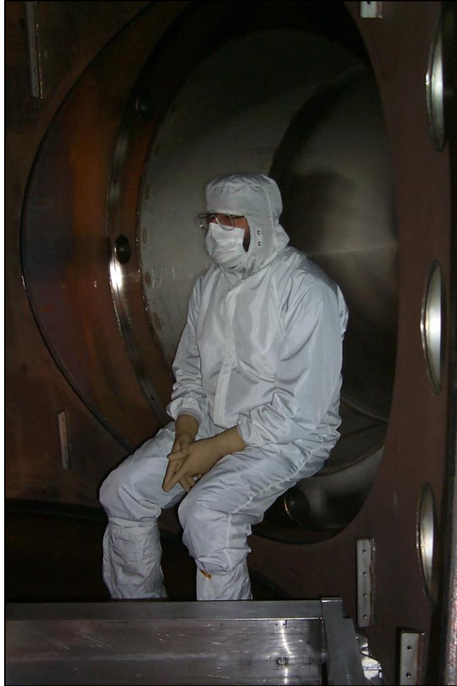
Taking a break during installation of the optics assembly at the LIGO Hanford Observatory in 2000.
